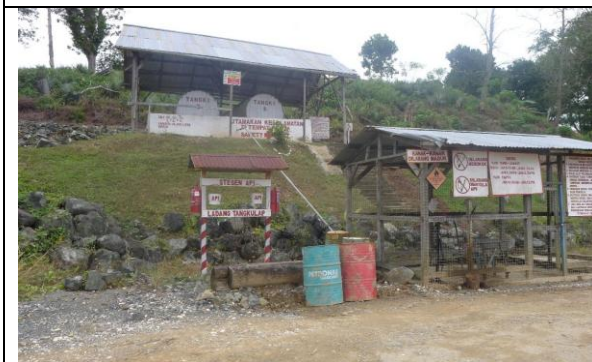
Storage and containment of diesel tanks
